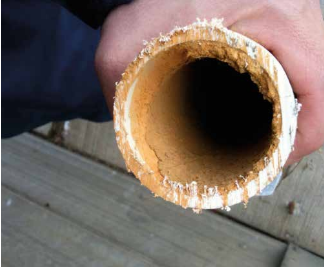
Iron and manganese build-up inside of a water line.
