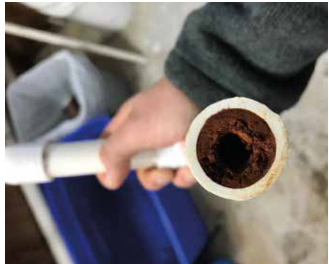
Iron build-up inside of a drinker line.
